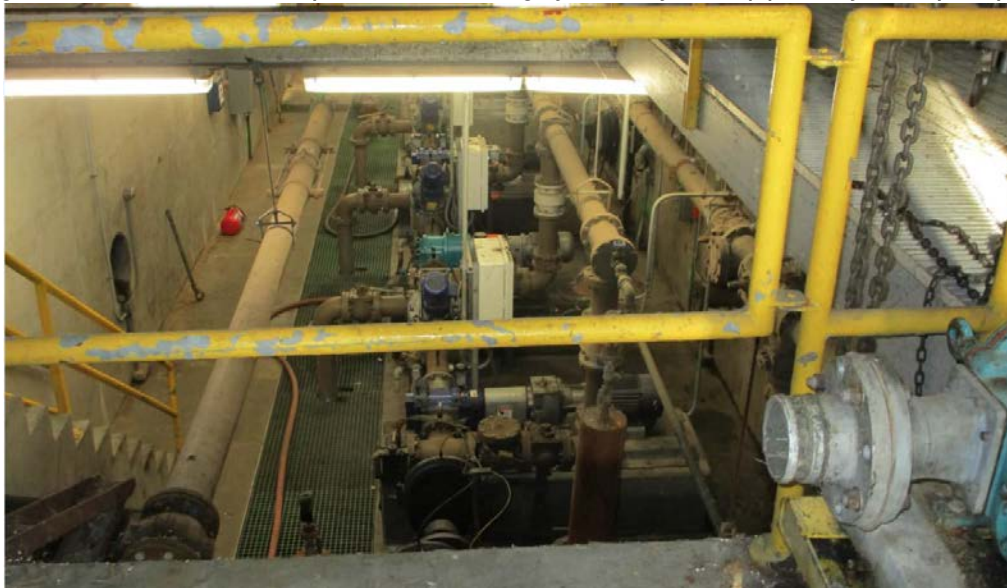
Figure 5 – Existing Combined Sludge Pump Gallery
