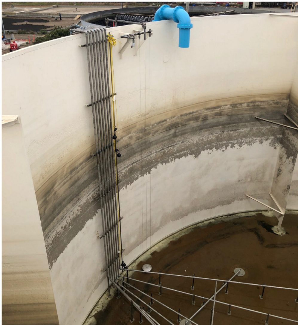
Image: Stainless steel air delivery piping on pipe tray
