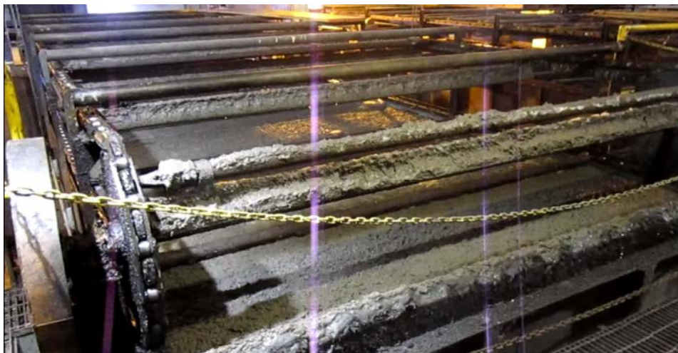
Figure 1: Existing DAF Unit
