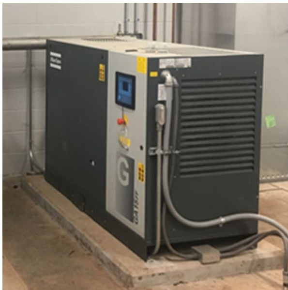
The compressor can be located indoors for weather protection and ease of maintenance in a climate-controlled environment
