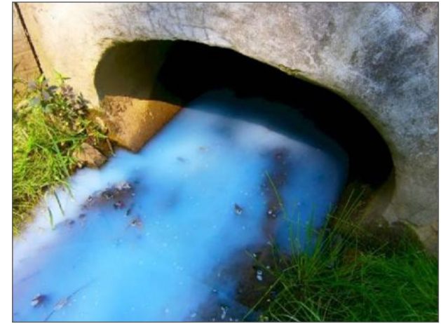
Illicit Discharge Prince William County, VA
