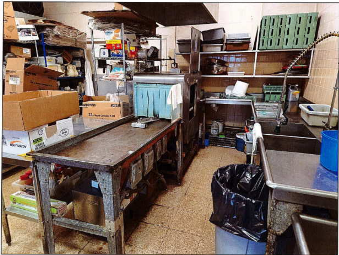
Photo of existing dishwasher which was originally installed in 1969. The equipment at that time was used and many believed it came from a ship.
