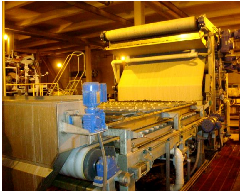
Two-Meter Belt Filter Press
