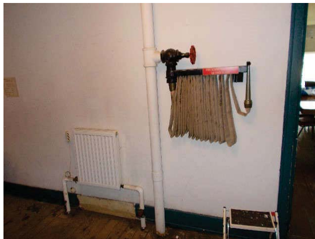
Hose rack located on 2 nd floor
