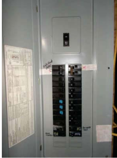
Photo 1 - Panel in basement
