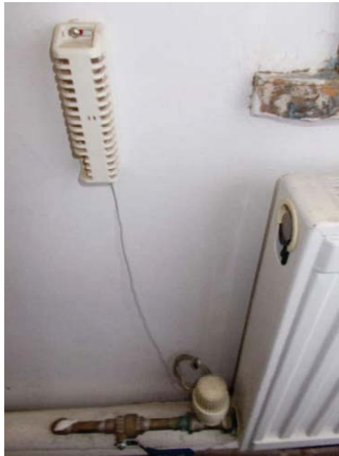
Remote temperature sensor installed on exterior wall.
