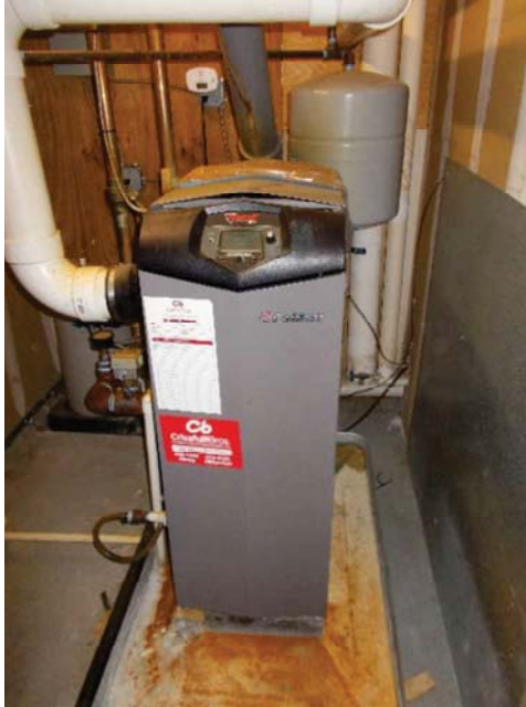
Gas-fired condensing boiler on 3 rd floor
