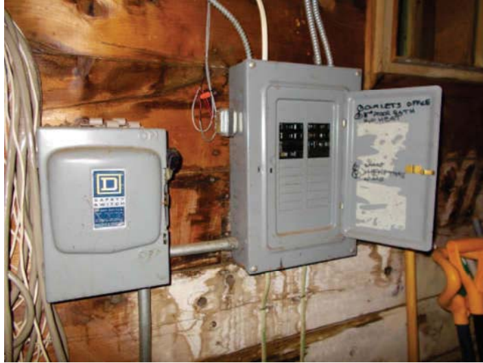
Photo 4 – Attic panel and disconnect switch
