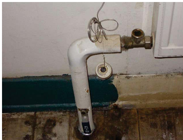
Broken actuator at thermostatic radiator valve
