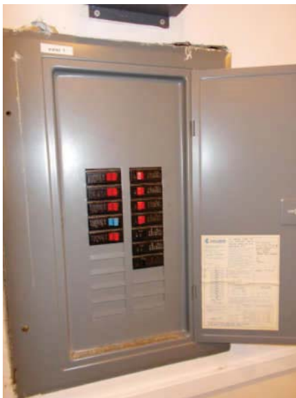
hoto 1 - Panel 1 on first floor
